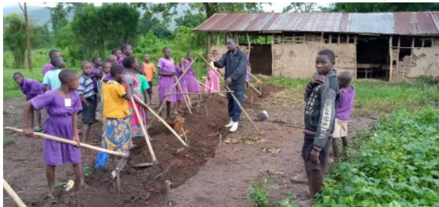
At Kisojjo school Godfrey Kisakye demonstrates how to use the A frame to dig contour ditches. The old, temporary classrooms are in the background.
